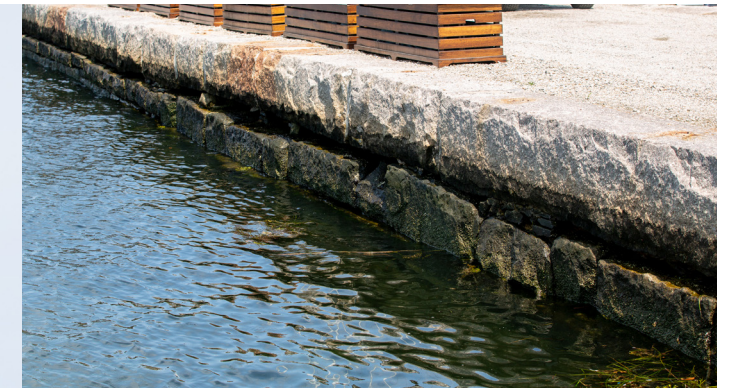
A granite capstone running the length of the seawall creates a unified look, but the wall base was built over time using varied construction techniques; today, more than 40 percent of the wall is in poor condition. Inset above: The leveling course just below the capstone has deteriorated, making the wall uneven.
